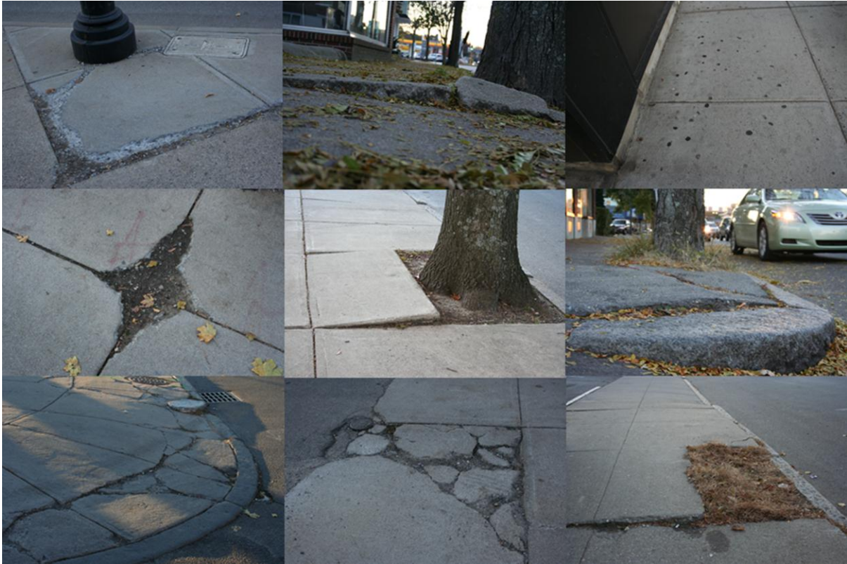
Figure 3-26: Numerous Damaged Sidewalks on Main Street
